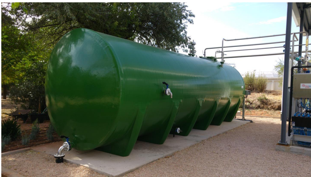
Figure 4: Anaerobic Reactor (40 m 3 )
