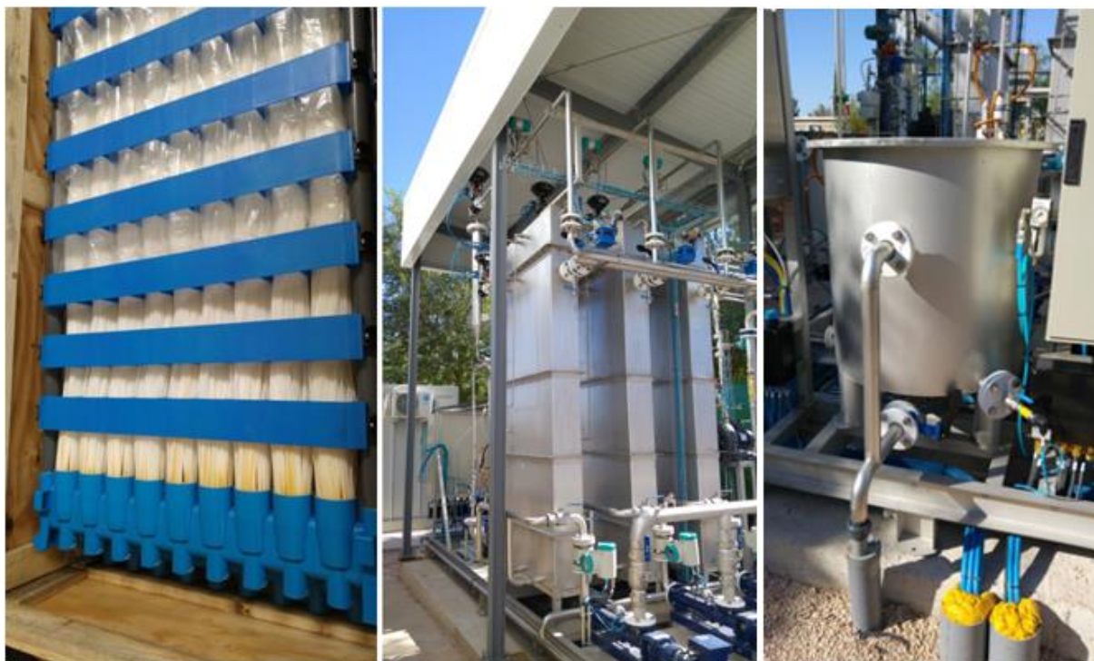
Figure 5: 3 Membrane tanks (PURON®, KMS, 41 m 2 filtration area/module, Ultrafiltration (0.03 µm)) and CIP tank
